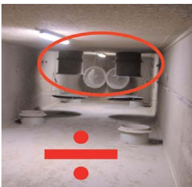
Partial purification established incorrectly.
