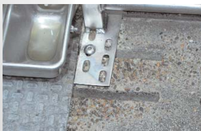
Corrosion of slatted floor in a pen floor treated with an impregnation product.
